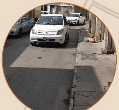
Lack of proper paving
