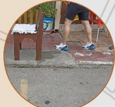
Lack of cohesion in the paving of the sidewalks
