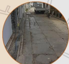
Lack of proper paving
